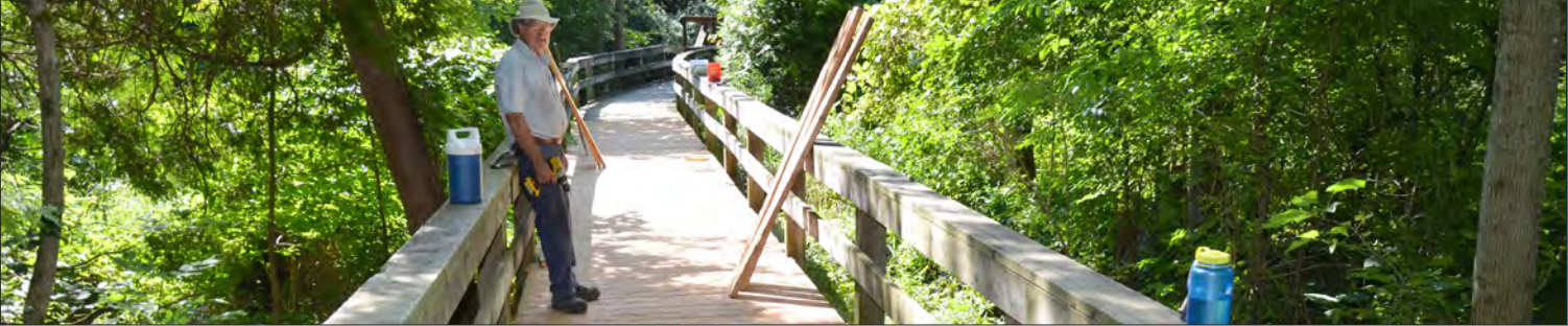
ABCA Field Services Staff Tony Drinkwalter replaces boards at Bannockburn Conservation Area.
