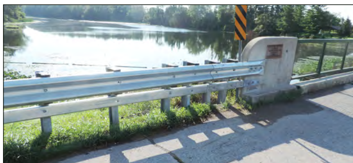
Replacement of hub rails at Morrison Dam, with a beam guiderail system, was one of the dam projects completed in 2016.
