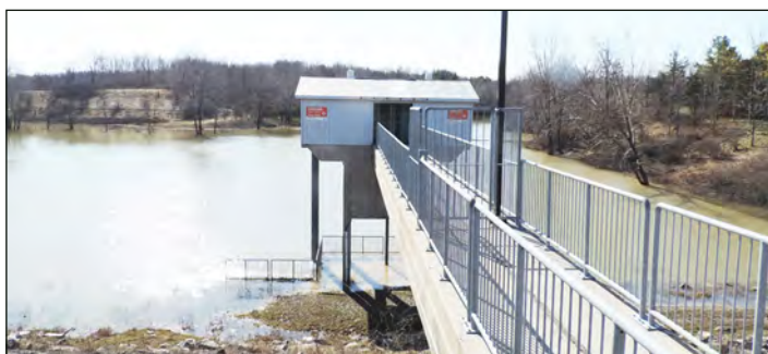
A safety review for Parkhill Dam (above), was started in 2015 and finished in 2016. A safety review was also completed for Morrison Dam.
