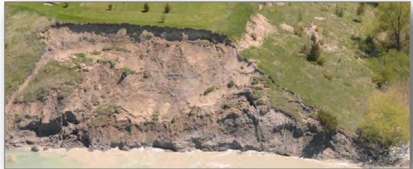
Slope failure along the Lake Huron Shoreline.
