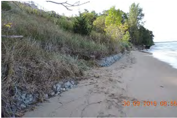
Insufficient materials were along some areas.
