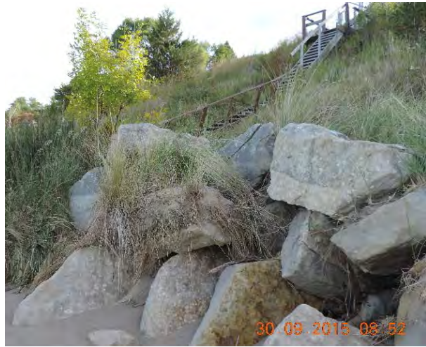
Randomly dumped stone at the toe of the steep slope.
