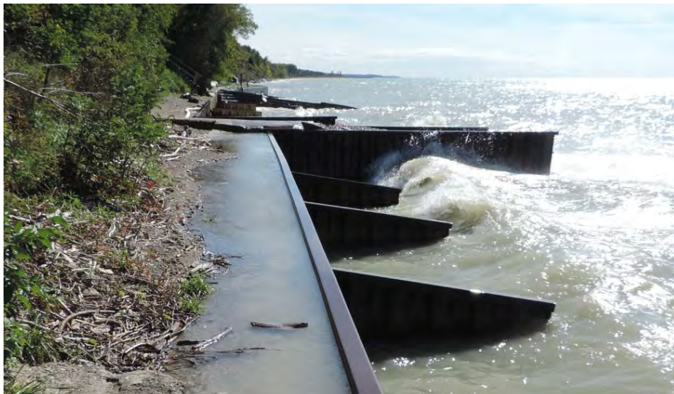
Wave Overtopping and ponding behind structures.
