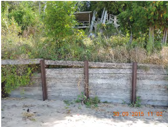
Deteriorated wooden frames.
