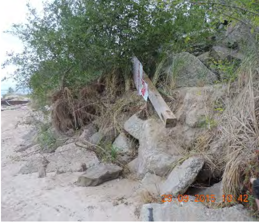
Dumped concrete rubble and stone.
