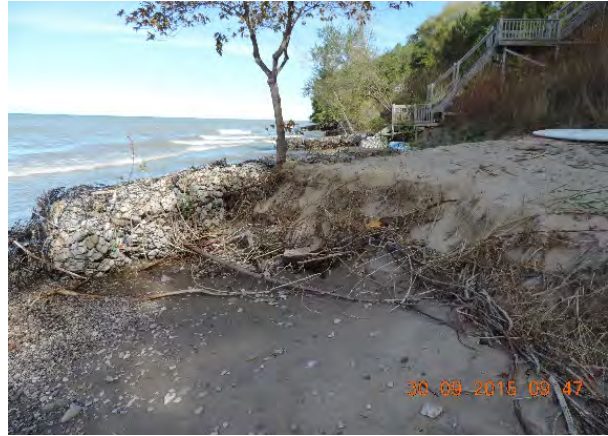
Outflanked and deteriorated gabion baskets.
