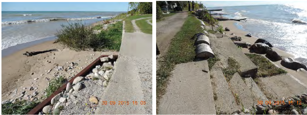
Figure 7.7: Drysdale Beach Road with development located along the toe of the bluff.
