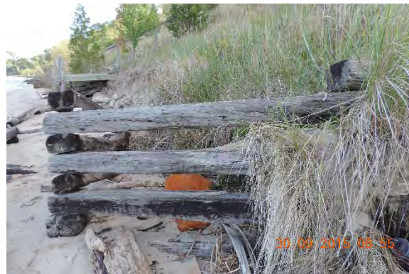
Deteriorated structures, emptied of materials.
