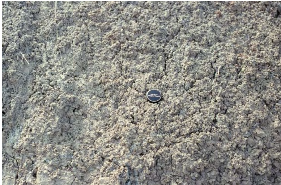
Figure 4: Weathering of till in cohesive bluffs, St. Catharines, Lake Ontario: a) bluff toe - wave erosion has removed weathered till in the right foreground and expansion cracks and fissures are just appearing. In the background small slumps have taken place in weathered material aided by snowmelt in the spring; b) drying of the surface layer in the summer produces a 'popcorn' surface of weathered silt and clay that is easily removed during heavy rains.
